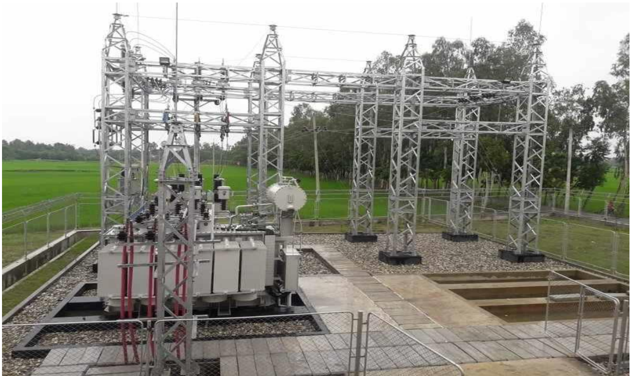
33/11KV, 10/14 MVA Sub-Station
